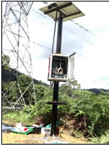
Fig. 7. Communication pole at site
