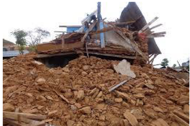
Fig. 3. Collapse of stone masonry in mud mortar building in the study area due to Gorkha Earthquake (Source: Santosh Lama, ward 3 beneficiary)
