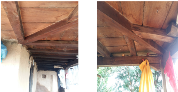
Fig. 12. Proper joint connections in the house that help to prevent the building from collapse
