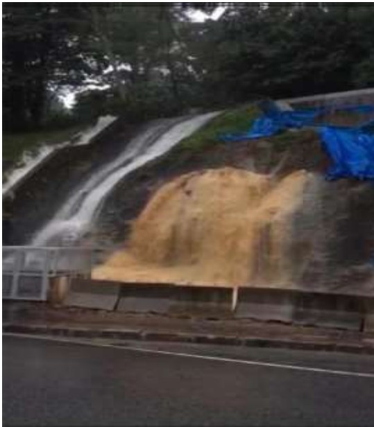
Fig. 3. A Slope failure adjacent to USM Hostels.
