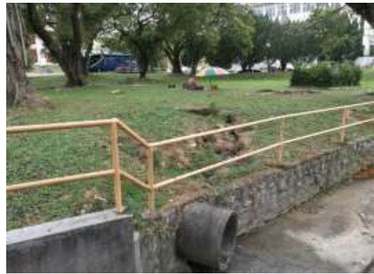
Fig. 9. Soil subsidence due to the water flow at USM, Penang.
