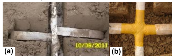
Fig. 11. VCM-MT using airtight membrane and horizontal perforated tubes (Long et al., 2011); (a) Connection of PVDs to horizontal flexible pipe and (b) Connection of horizontal and longitudinal pipe.
