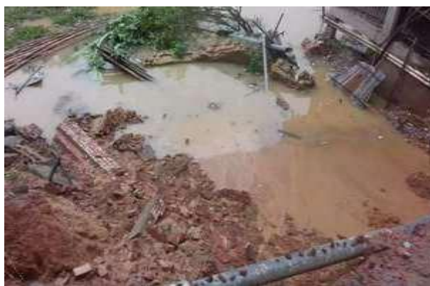
Photo 1. Water pipe in spot of Landslide
