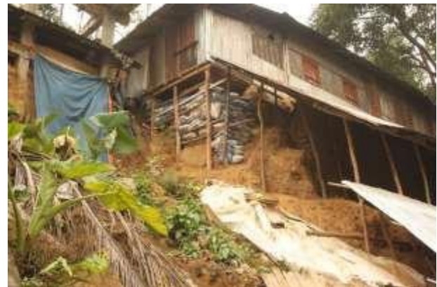
Photo 4. A vulnerable house at the steep slope
