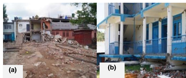
Fig. 5 (a). Damage school in Kathmandu, that at the time of the visit was being demolished (b) Collapsed school near Chautara
