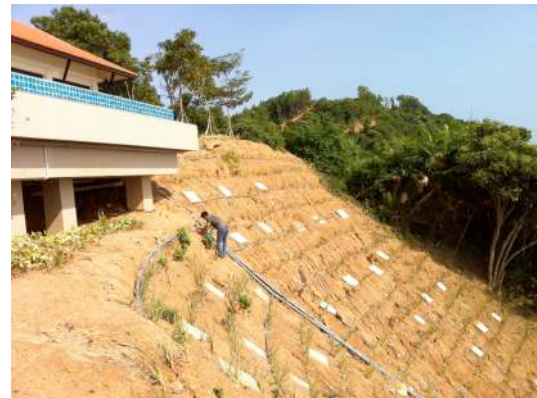
Fig.16. Auto irrigation system.
