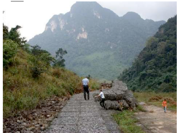
Fig. 4. The failure a slope on Ho Chi Minh high way (Van and Truong 2011)
