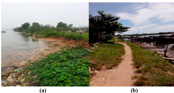
Fig. 1. (a) Erosion on the river at Gia Do commune; (b) Erosion at the dyke system at Quy Ha commune.
