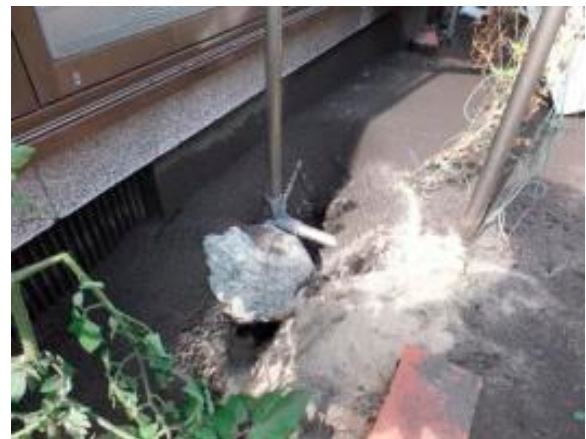
Fig. 3. Sand boiling in a house in Minami ku, Kumamoto
