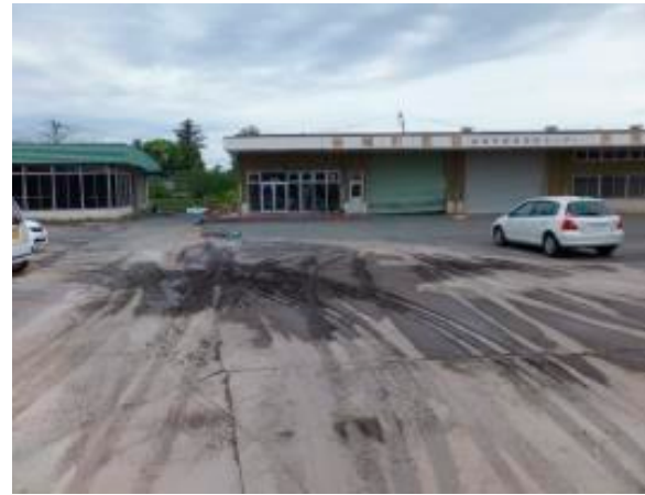
Fig. 2. Sand boiling at a parking lot of JA-Kamimashiki
