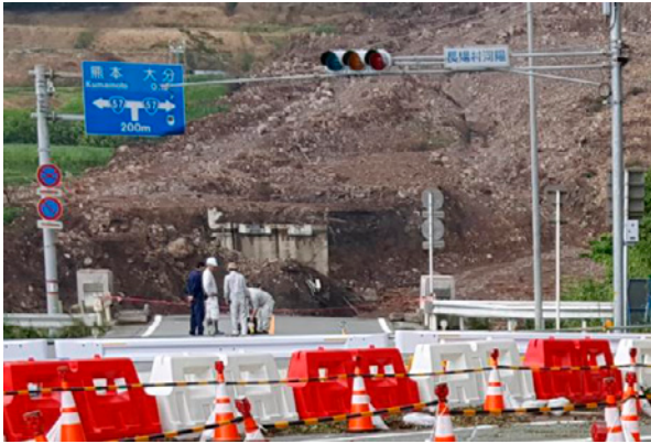
Fig. 2. Bridge collapse and landslide.
