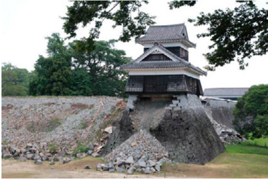
Fig. 18. Photograph of Inui Yagura (right: 2003 reconstruction), a wooden two-floor three-story turret that was rebuilt in 2003. Inui Yagura foundation was partial collapse in the middle of the stone wall. (photo by T. Ohsumi, taken July 20, 2016)
