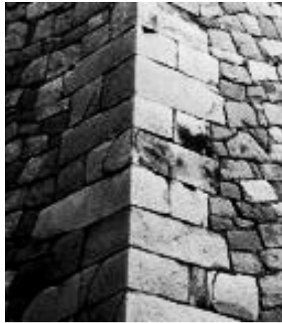
Fig. 4. Example of the Sanki-tsumi construction method at Nagoya Castle, Aichi Prefecture, (photo by T. Ohsumi, taken in 1990).
