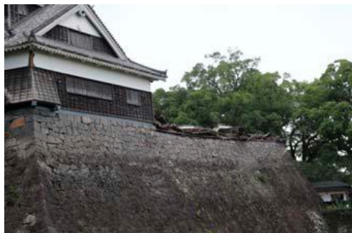
Fig. 14. Photograph of Tsuzuki Yagura taken from Kato Shrine. Unlike Uto Yagura, this turret was not reinforced to be earthquake resistant, and collapsed after the earthquakes (photo by T. Ohsumi, taken August 11, 2016).
