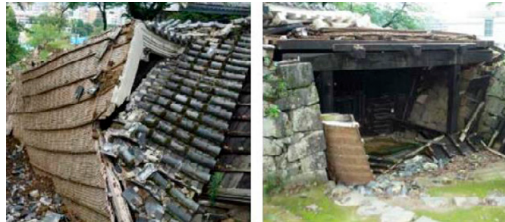
Fig. 21. Photograph of Akazu-no-mon, which was designated as an important cultural property, was heavily damaged by the earthquakes (courtesy of Prof. K. Meguro, taken Oct. 26, 2016).
