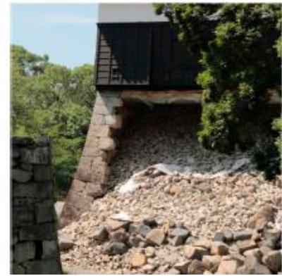
Fig. 8. Photograph of the stone wall of Bagu Yagura (1966 reconstruction), constructed using the Sangi-tsumi method. (photo by T. Ohsumi, taken Aug. 11, 2016)
