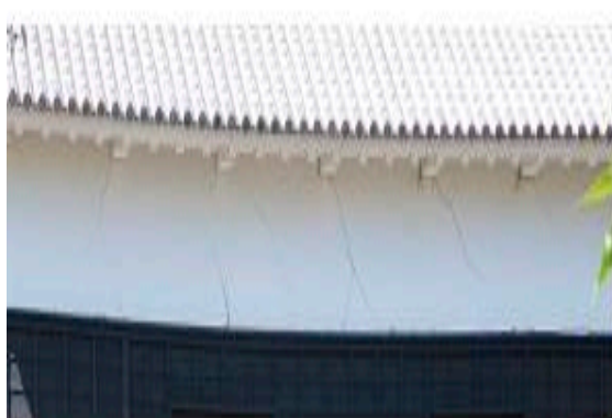
Fig. 30. Photograph showing enlargement of foundation settlement caused the white wall at Bagu Yagura (photo by T. Ohsumi, taken July 20, 2016)
