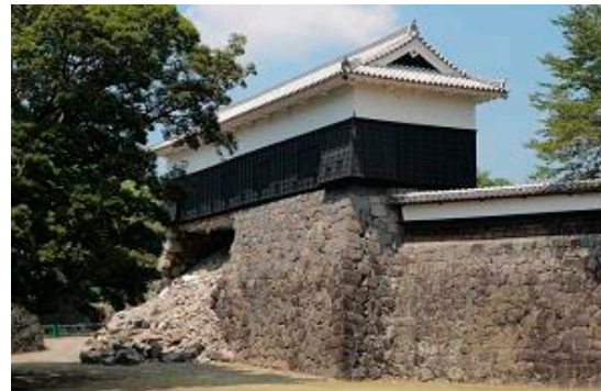
Fig. 28. Photograph of Naga-kabe and Bagu Yagura-dai (1966 reconstruction) (photo by T. Ohsumi, taken August 11, 2016)
