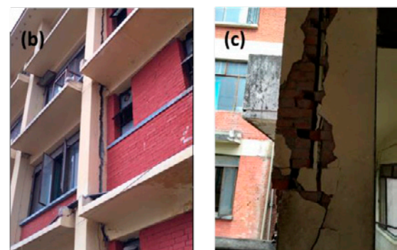
Fig. 15. (a) Soft story collapse of school in Chautara (b) and (c) structural damage to hospitals in Kathmandu.
