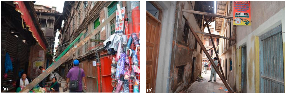
Fig. 3. Iron and wooden frames are used to give support on the narrow streets of south Durbar square. Clusters of old aged, renovated buildings combined with RCC buildings are distributed along this narrow streets. Most of the houses remain intact from support interconnected with each other.
