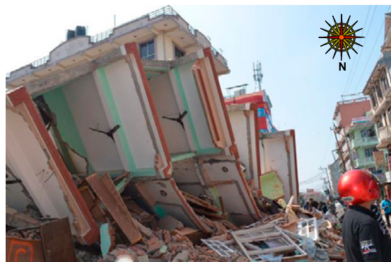
Fig. 23. Topped RCC building in Gongabu area, Kathmandu. Tilted towards the south direction.
