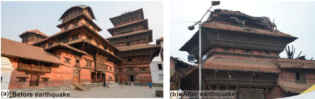
Fig. 11. Nyatapola (Basantapur tower) (a) inner premises of the former royal palace, a recent museum (Courtesy: Wikipedia) and (b) damages occurred at the roof and adjacent parts.
