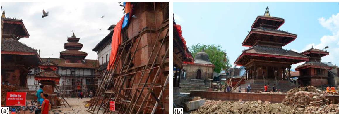
Fig. 14. Damages at (a) Hanumandhoka and (b) around Hanumandhoka.
