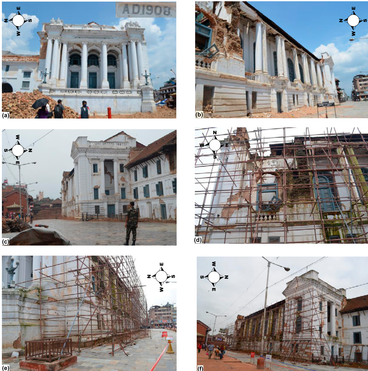
Fig. 10. British Government constructed this White Palace in 1908 AD. It was extensively damaged during the quake. Photographs (a), (b) and (c) represent the survey immediate after the main shock and aftershock in the month of May, 2015 while photographs (d), (e) and (f) show the rod framework supports on both sides of the palace to protect from immediate collapse. The photographs were snapped during the second survey on July 21, 2015.
