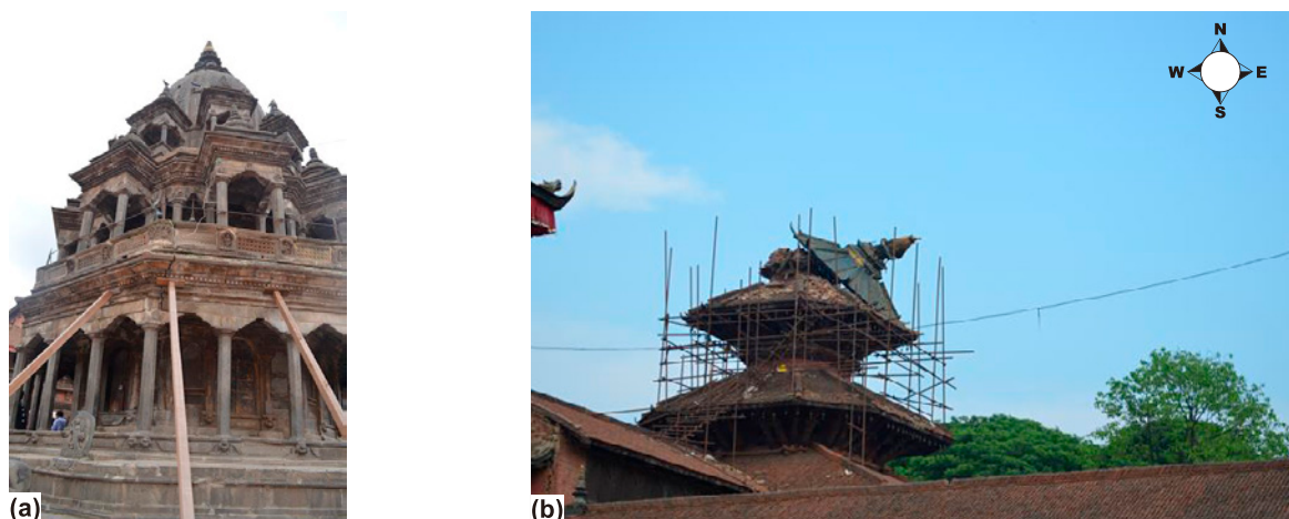
Fig. 17. Damages in Patan Durbar Square (a) Chyasim Deval Krishna Mandir and (b) toppling of the temple top in the east direction.
