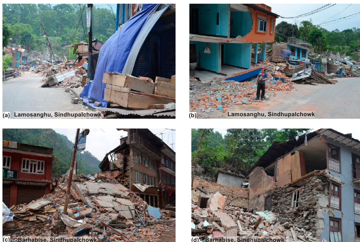
Fig. 8. Damages appeared along the Araniko Highway in Sindhupalchowk district: (a) Tilted poles and rubbles of houses can be seen at Lamosanghu area (b) Soft-story failure in RCC building at Lamosanghu, (c) Total collapse of concrete building at Barhabise, and (d) Debris of houses and severely damaged stone wall house at Barhabise.
