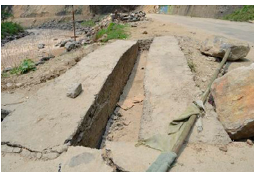
Fig. 28. Culvert and retaining structure on the bank of the of the river along the highway was severely affected.
