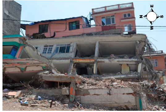
Fig. 21. Topped RCC building at Anand Nagar, Sitapailai, Ringroad, Kathmandu. Tilted towards the east direction.
