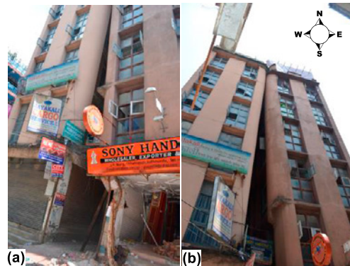
Fig. 25. Tilted RCC building at J.P. Marg, Kathmandu. Tilted towards the east direction
