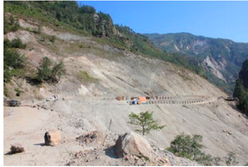
Fig. 31. Deep-seated landslide of Daklan affecting Arniko Highway. View to S.
