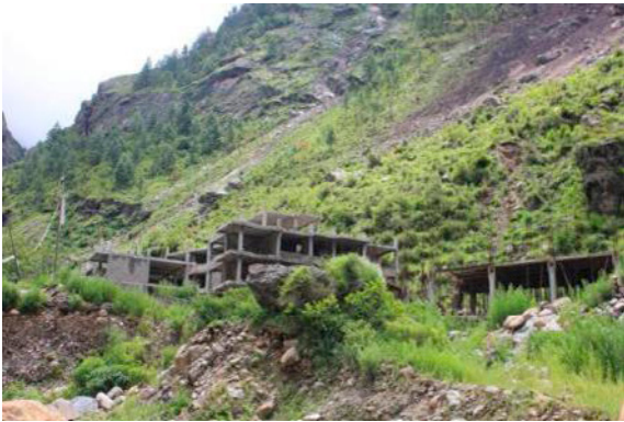
Fig. 19. Buildings of Rasuwa Gadhi Hydropower Project damaged by rock fall. View to E.
