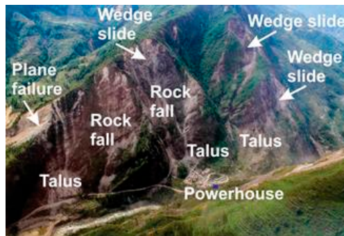
Fig. 29. Rock falls and shallow slides developed above the Upper Bhoté Koshi Powerhouse. View to SE.
