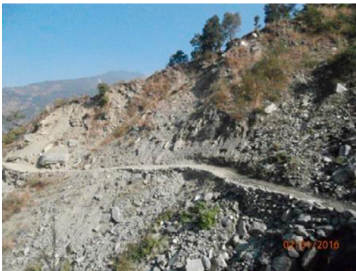
Fig. 17. Dharna colluvial slide affecting Dundure-Dhading Besi road.
