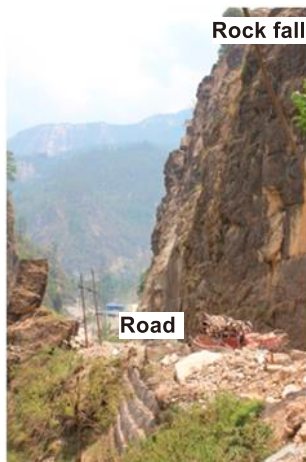
Fig. 28. Cliff south of Chaku, where Arniko Highway is suffering from rock falls. View to N.
