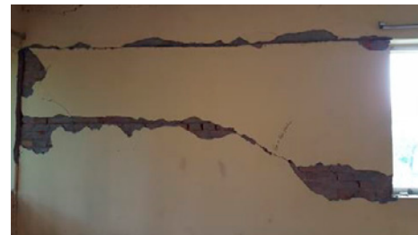
Fig. 7. Cracks seen in masonry infill wall.
