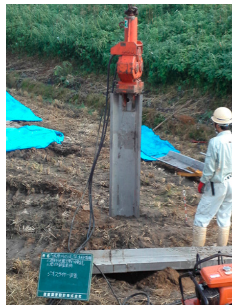
Fig.7 A weighted vibrator is used to penetrate the Geoslicer to the ground.
