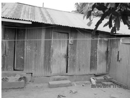
Fig. 10. Housing materials used in the study area; Corrugated Iron sheets on roof and walls; mud floor.
