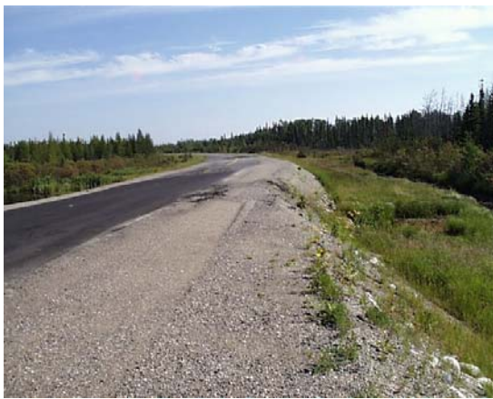
Fig. 2 Road embankment in Northern Manitoba showing signs of lateral movements and differential settlements (courtesy of Manitoba Transportation and Government Services)
