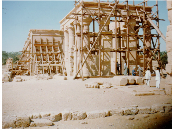
Fig. 12 Failure of Hepies Temple due to groundwater rise
