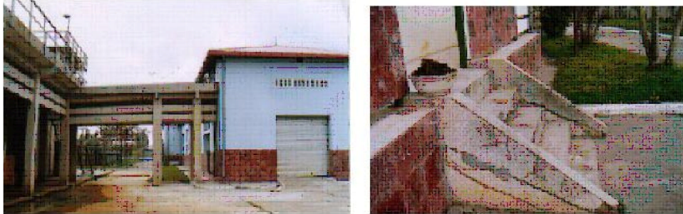
Fig. 8 Land subsidence at the Phap Van water plant: (i) Left: Differential settlement at the sedimentation basin; (ii) Right: Cracks of the steps to the office buildings
