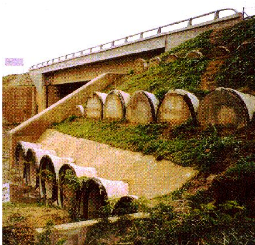
Fig. 9 View of the three rows of concrete pipes aimed at decreasing the weight of the access embankments of the bridge over the Drader river
