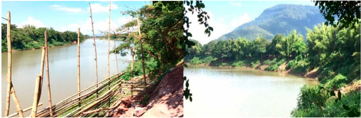
Fig. 6. Photos of Xedon Riverbank erosion at the outer curve.
