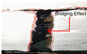
Figure 10. Crack width - first crack
