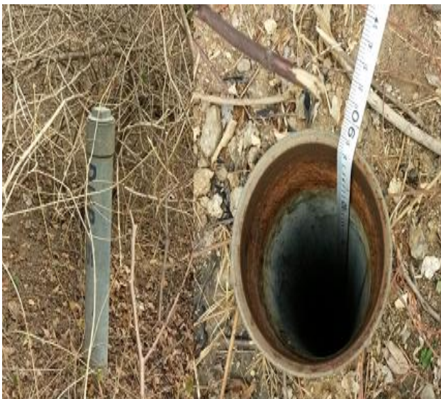
Fig. 5. Observation well for ground water level
