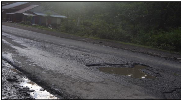
Figure 2. Road damage due to trucks that often pass
