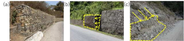
Figure 3. Example of damage; (a) No major damage; (b) Partial deformation; (c) Collapse
