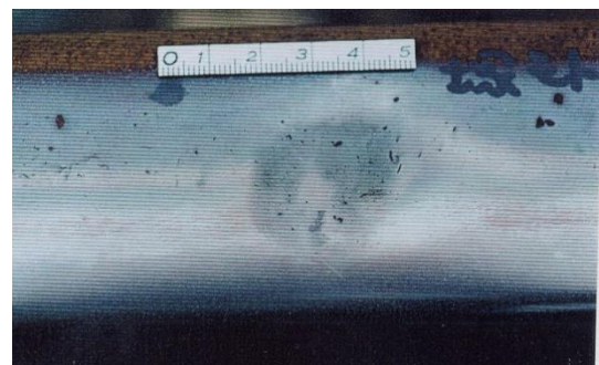
Figure 4. Typical RCF defect “Squat” called in UK and rail surface shelling called in Japan
