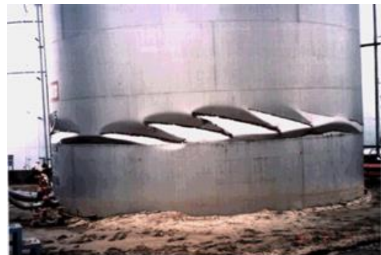
Figure 10. Diamond-shape buckle of a sidewall in a small AST in Kobe at the 1995 Kobe Earthquake (Courtesy of National Research Institute of Fire and Disaster, Japan)
