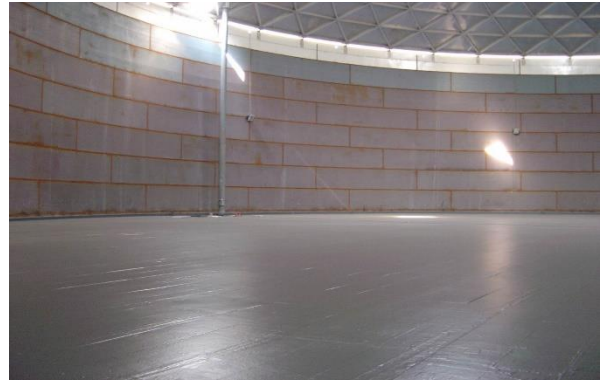
Figure 18. Unsinkable FRP floating roof (Courtesy of HMT Inc.)
