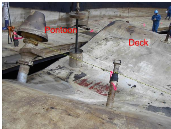
Figure 16. Deck plate and pontoon of a sunk single-deck floating roof of a 100,000 m 3 crude oil storage tank at the 2003 Hokkaido Earthquake
