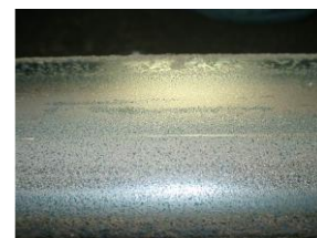
Figure 29. State of top surface of rail
