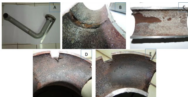
Figure 1. (a) Visual condition of the corroded tubing, (b) section of failed tubing, (c) corrosion at the weldment and straight pipe, (d) condition of the elbow pipe before cleaning, and (e) pit revealed after cleaning
