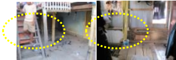
Figure 3. Illustration of the addition of space to the residence without a good planning on the structure and construction of the residence
