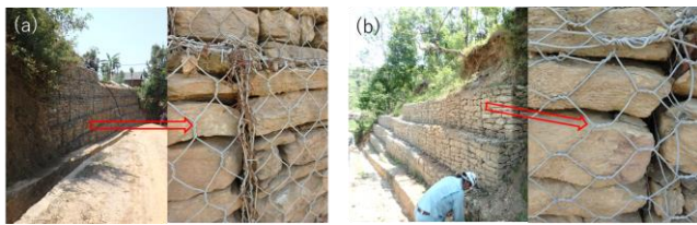
Figure 8. Trial construction of a gabion-based retaining wall [7]. The direction of the turtle-shell-shaped wire mesh had not been considered. (a) Mesh line is vertical. (b) Mesh line is horizontal
