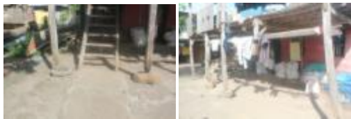
Figure 4. Illustration of the insecure residence construction in Letta village because of the live/dead loads and aged wood material.
