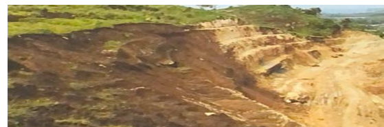
Figure 1. Landslide location at STA 1+075 – 1+100
