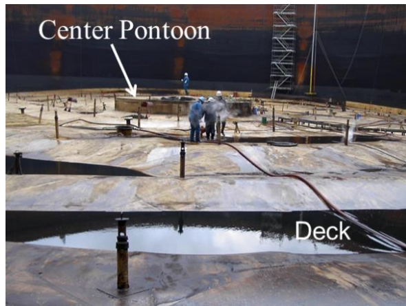
Figure 15. Deck plate of a sunk single-deck floating roof of a 100,000 m 3 crude oil storage tank at the 2003 Hokkaido Earthquake
