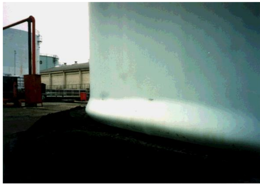
Figure 11. Elephant foot bulge of a sidewall in a small AST in Kobe at the 1995 Kobe Earthquake (Courtesy of National Research Institute of Fire and Disaster, Japan)
