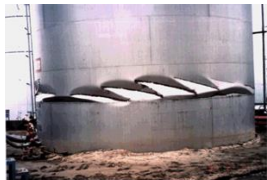
Figure 10. Diamond-shape buckle of a sidewall in a small AST in Kobe at the 1995 Kobe Earthquake (Courtesy of National Research Institute of Fire and Disaster, Japan)
