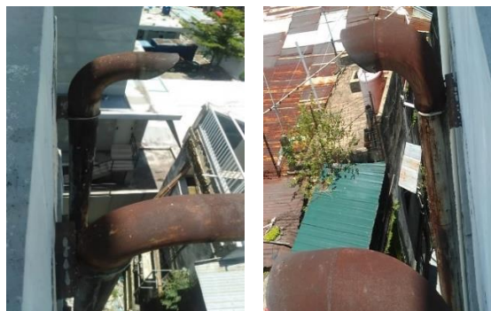
Figure 6. HVAC exhaust pipe in Makassar Bosowa Tower Parking building
